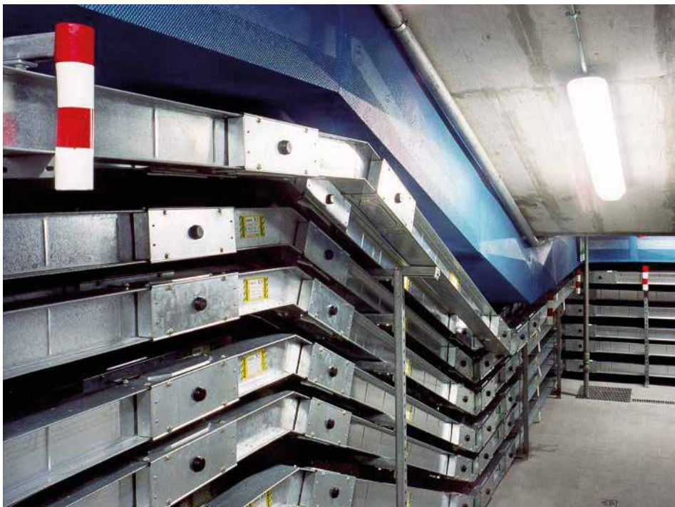
Example of high power distribution
