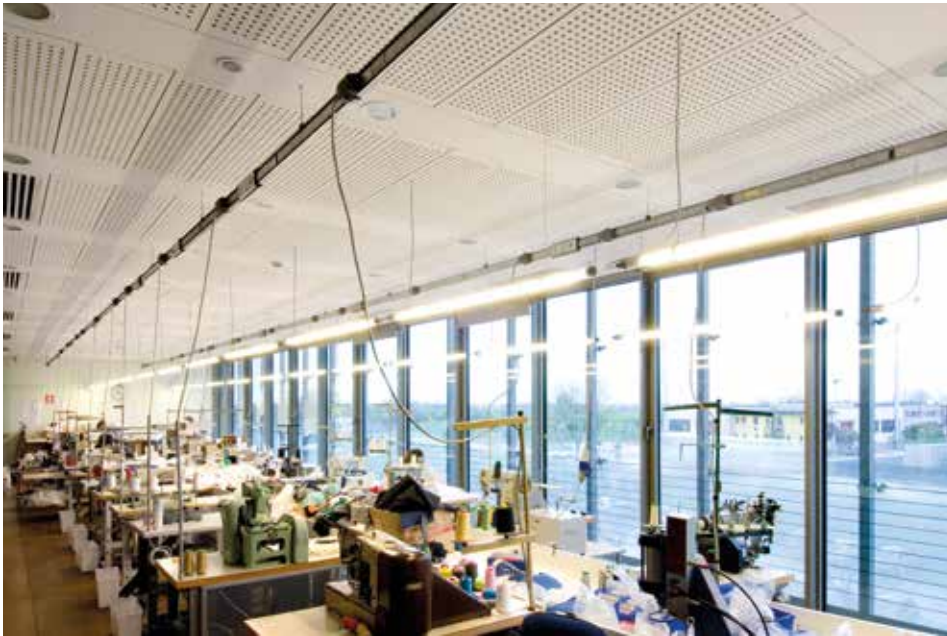
Example of lighting and small power distribution
